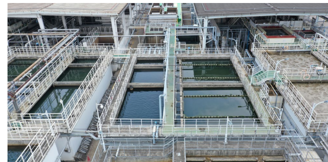
GAC-Toyota's sewage treatment station
